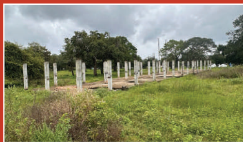
Construction of transit housing project in Mannar under a grant of SLR 400 million
